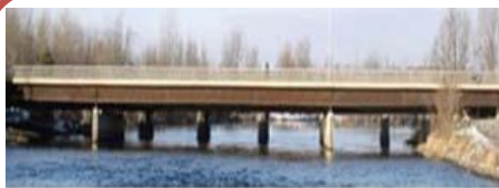
A Girder Bridge is usually built using: steel beams and reinforced concrete
